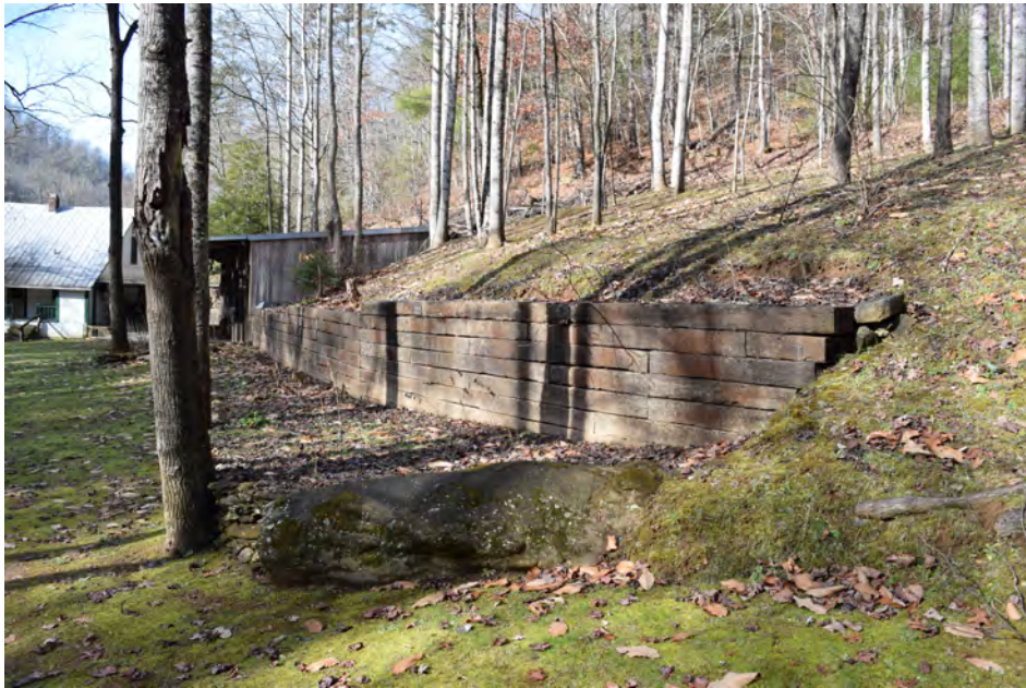
Retaining wall on north side of parcel, view to the northwest toward shed and house
