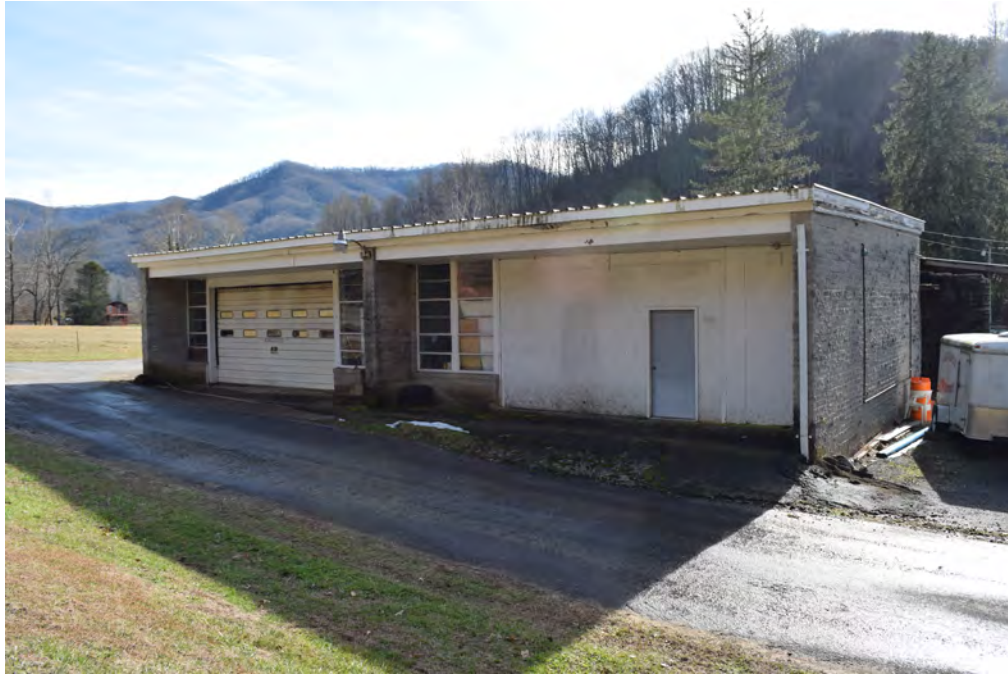
North elevation of the 1958 addition containing the two classrooms, view to the southeast
